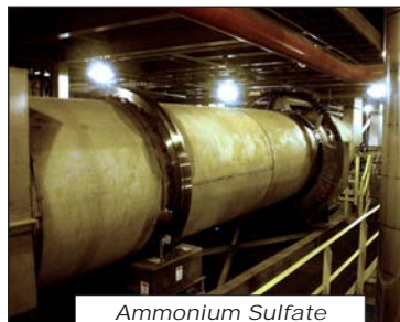
Ammonium Sulfate Dryer
