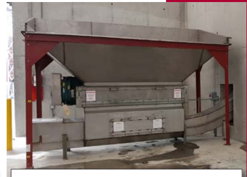
300tph System in fixed configuration
